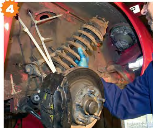
4 Removing the front suspension isn't as easy as the rear. The top and bottom mounts are easy to undo but the shock won't pull out of the top wishbone without removing it.
